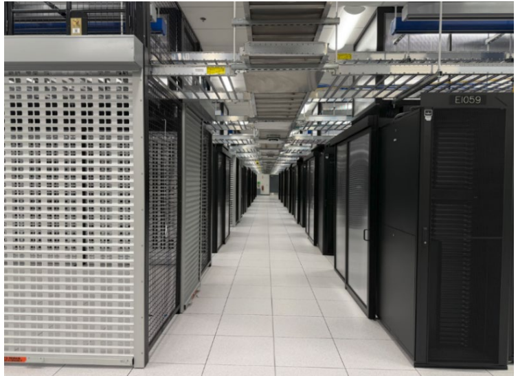
Data hall inside US Signal
