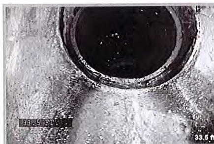
Green dye seen coming from an illicit connection when dye testing
